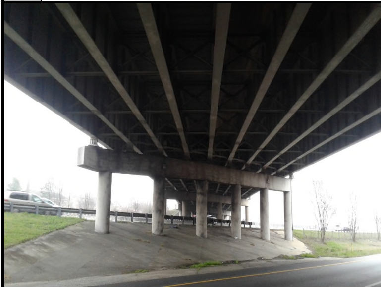
3 View of the underside of the bridge. Shows metal decking, steel beams, and concrete piers.
