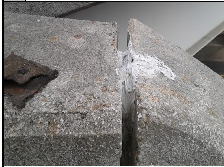
4 The gray caulking tested negative for asbestos via PLM and TEM analysis.
