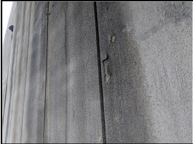
5 The expansion joint material located on the boundary wall tested negative for asbestos via PLM and TEM analysis. The textured material tested negative for asbestos via PLM analysis.
